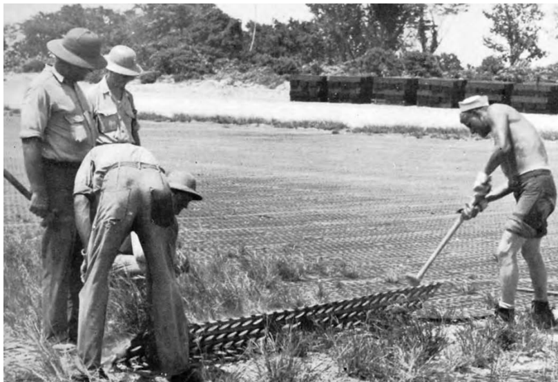
Men from the 57 th Construction Battalion lay Marsden mat for the construction of an airfield on Espiritu Santo.
